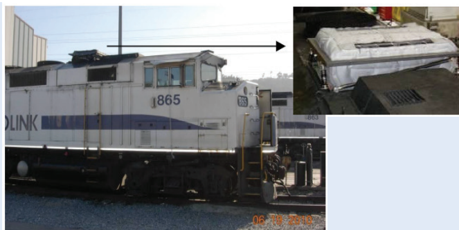
Figure 1: Compact SCR catalyst assembly installed in SCAX 865
